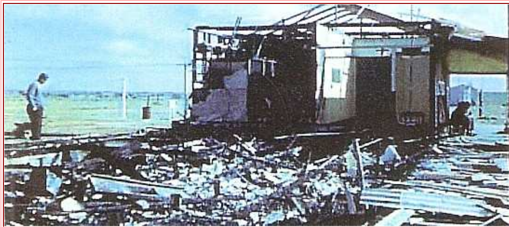
Fire in 1957 Most of the building was burnt to the ground. The section housing Aeradio was still standing. The radio equipment, after clean up, was recovered. (Photo ref. 6)
